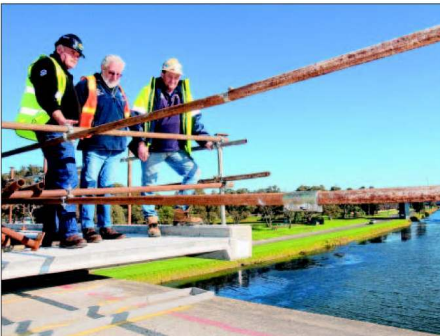
STALLED: CFMEU's Brendan Murphy, independent consultant Maurie Hill and civil organiser Adam Hall on the bridge.
